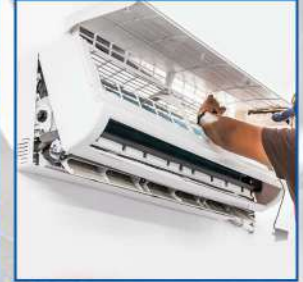
Air Conditioning Ventilation & Air Filtration Systems
