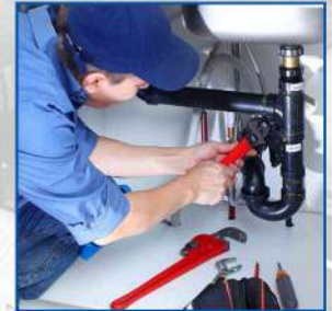
Plumbing & Sanitary Contracting
